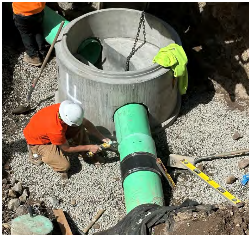
Figure 4- MCWD crew connecting to the existing stub-out at the downstream end of the project. This stub-out was installed as part of The Parcel Phase 1 construction.
