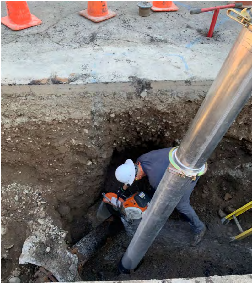
Figure 3- Cutting into the MCWD water main to re-align the pipe to avoid conflict with the new sewer main
