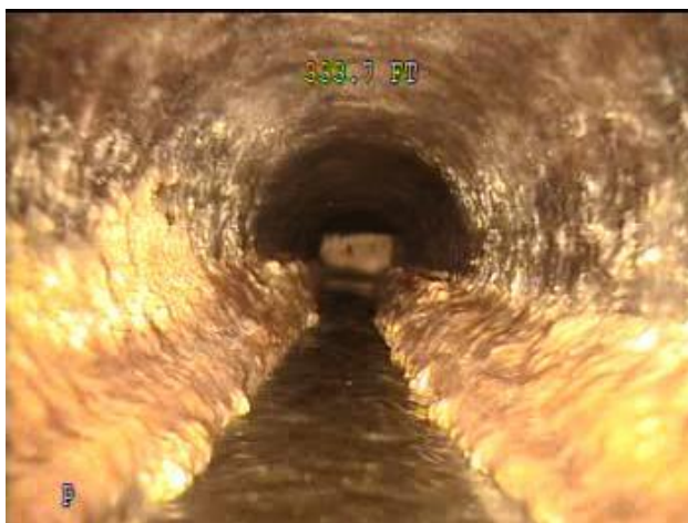
Sewer line in Mammoth starting to accumulate grease.
